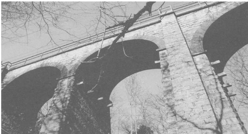
Figure 1. A typical example of structure to be identified: a masonry arch bridge. The geometrical shape can be correctly captured, different cortical construction materials can be mapped by visual inspection and boreholes can be used for fillings.
