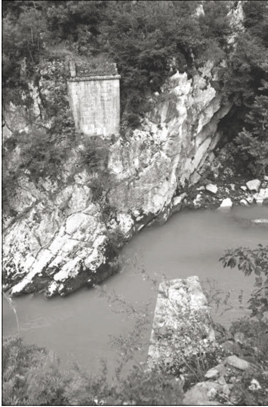
Fig. 4: The bridgehead along the Devrekani at Atköprü. Note the wall in the lower right of the picture, which is part of the bridgehead on the eastern side (©CAP).
