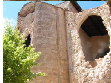
The apses before (top) and after (bottom) the 2009 L'Aquila earthquake
